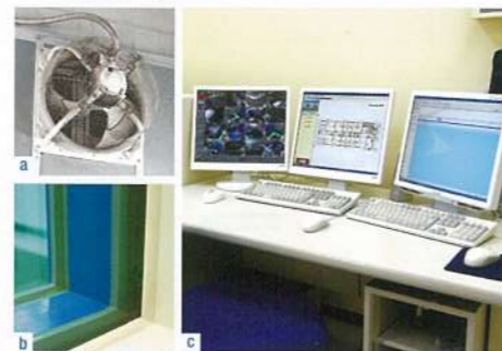
a/ Forced ventilation fan b/ Dual structure window consisting of bulletproof glass and fireproof glass c/ Central monitor room
